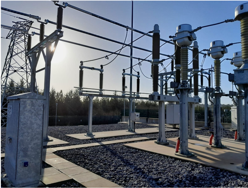
Figure 7: Typical 110kV Electrical Infrastructure
