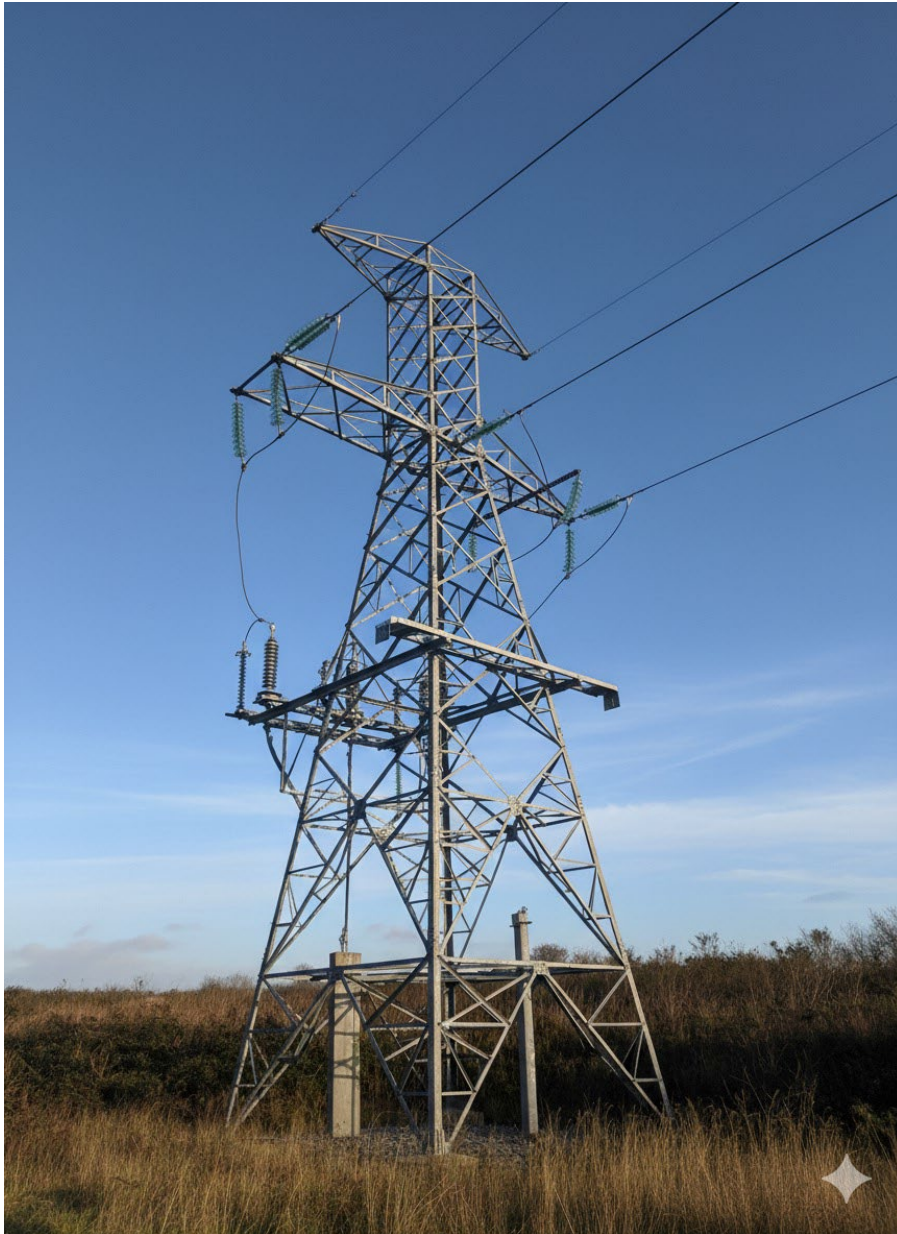
Figure 6: Cable End Mast
